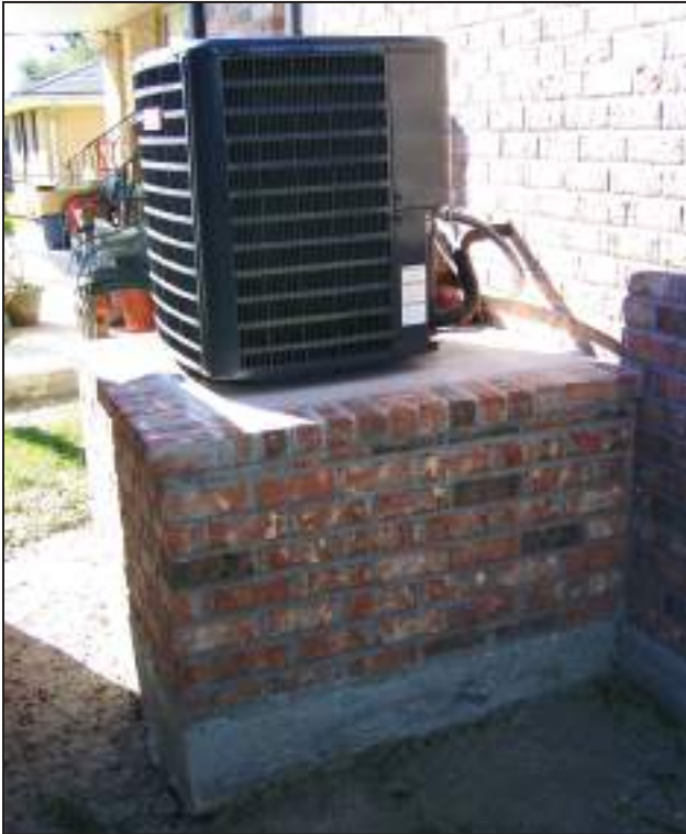
Figure 3-1. Air conditioning compressor elevated on a pedestal.
