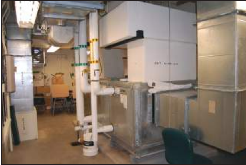
Figure 5-6. AHU with a separate chilled water coil (green labels) and hot water coil (yellow labels). The coils are within the unit and are not visible (Dagsboro, Delaware).
