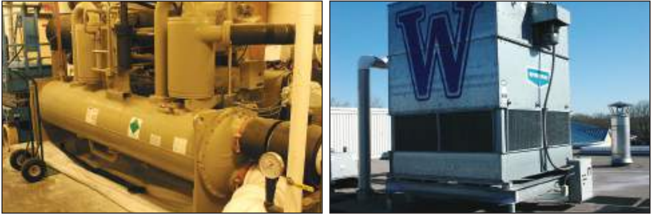
Figure 5-2. Indoor water-cooled chiller (left) with rooftop evaporative cooling tower (right) in Bridgeville, Delaware.
