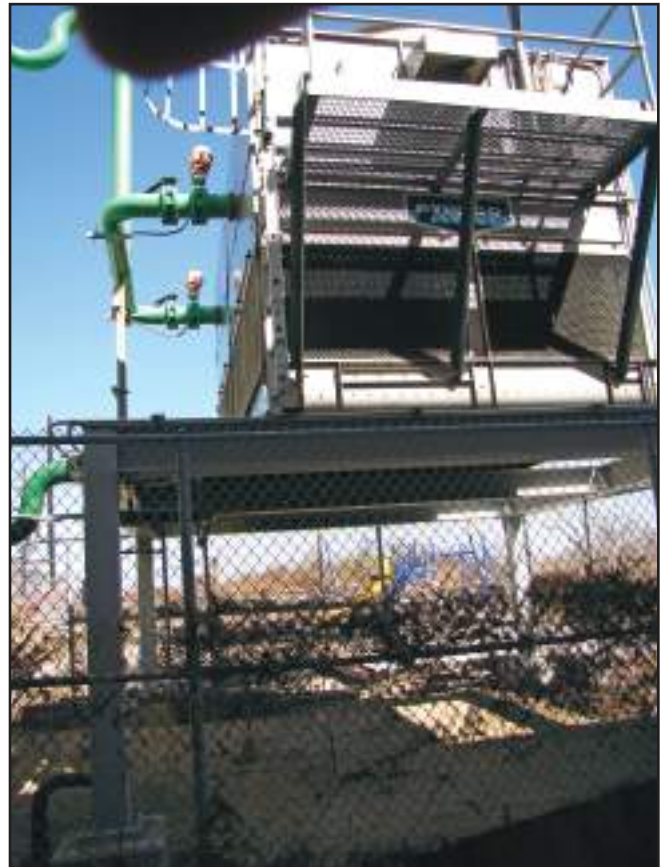
Figure 5-7. Cooling tower placed on an elevated frame (Hurricane Ike, Port Bolivar, Texas, October 18, 2008).
