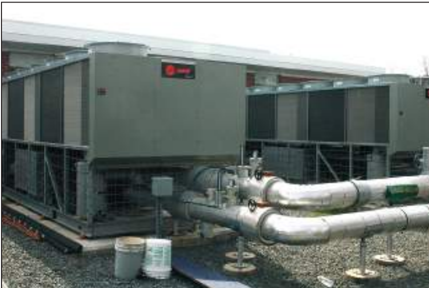
Figure 5-3. Air-Cooled rooftop chiller in Georgetown, Delaware.
