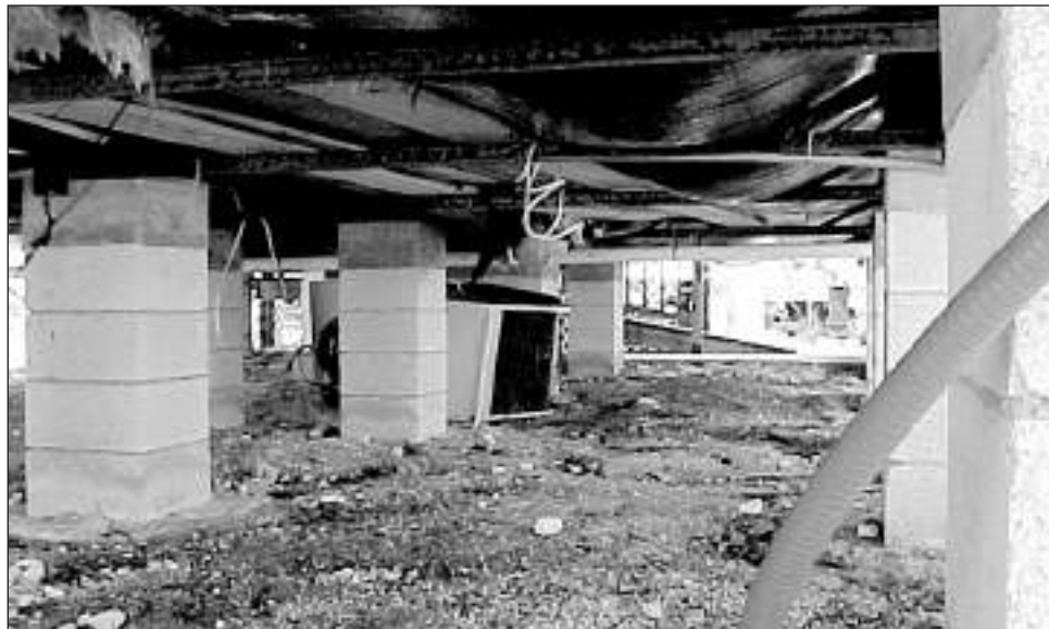
Figure 1-4. Reinforced masonry pier foundation system under a manufactured home installed after 1994 that performed well.
