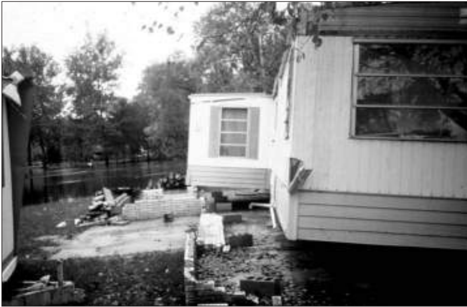
Figure 9-1. A home that was partially submerged and displaced from its foundation by hydrostatic forces. Although it appears the openings are too high, the bottoms of the openings are less than 1 foot above the top of the interior slab.
