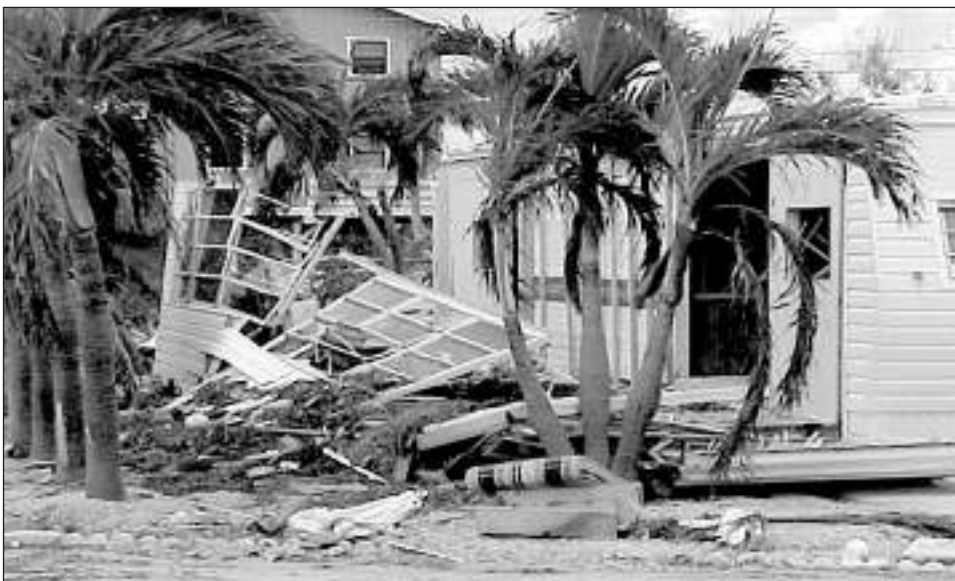
Figure 1-3. The addition to this manufactured home was destroyed, causing considerable damage to the rest of the home.
