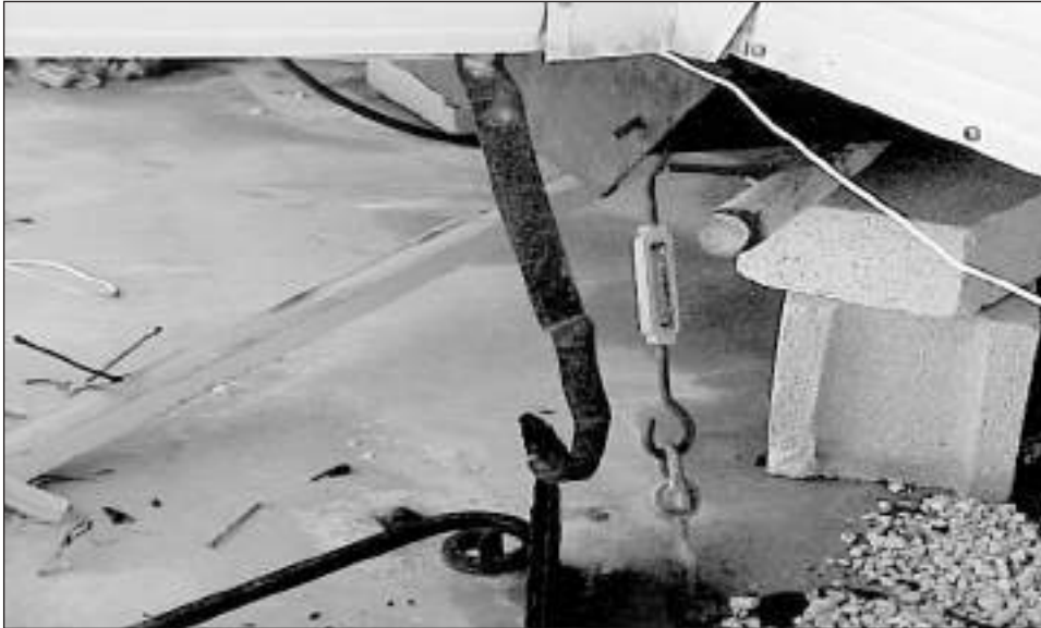
Figure 1-2. Inadequate turnbuckle anchor installed by the homeowner on this pre-1994 manufactured home, coupled with lack of elevation and an unreinforced foundation system, led to severe damage.
