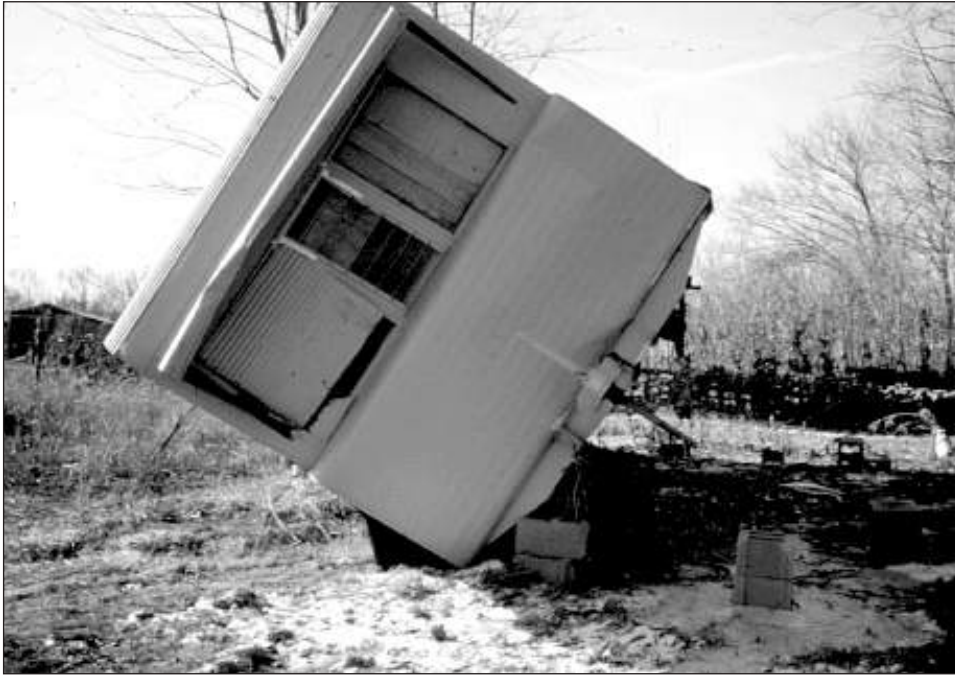
Figure 7-8. Failed foundation system that used masonry piers.
